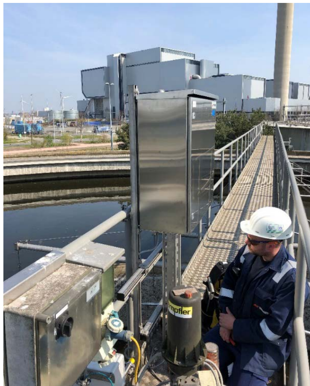
Figure 1: Sludge level sensor installation
